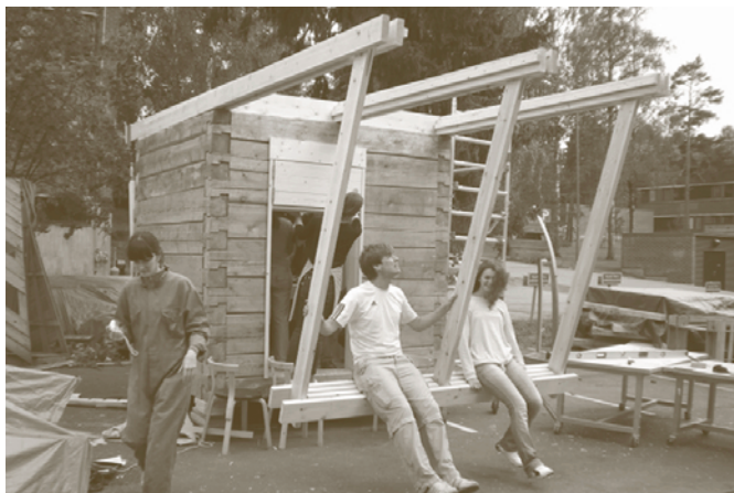
Amazement as the tension bars hold, the four person works and the roof hasn't ripped off!
