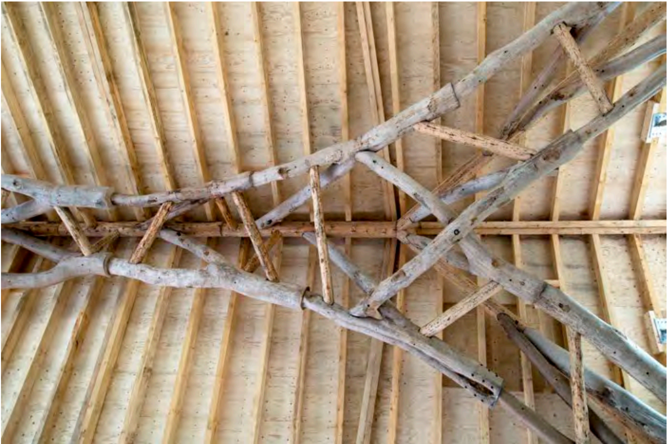
The Wood Chip Barn's robotically fabricated 'tree fork truss' is made of 20 distinct beech forks. Through digital design and fabrication tools the inherent form and structural capacity of the tree is employed directly. Completed in 2016
