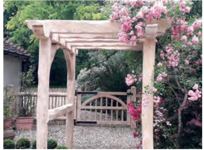
A newly installed rose draped pergola leads to a new gate and fence
