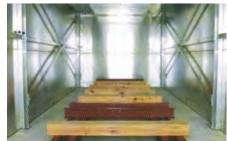
Interior of the kiln showing the heat exchangers and intermediate ceilings
