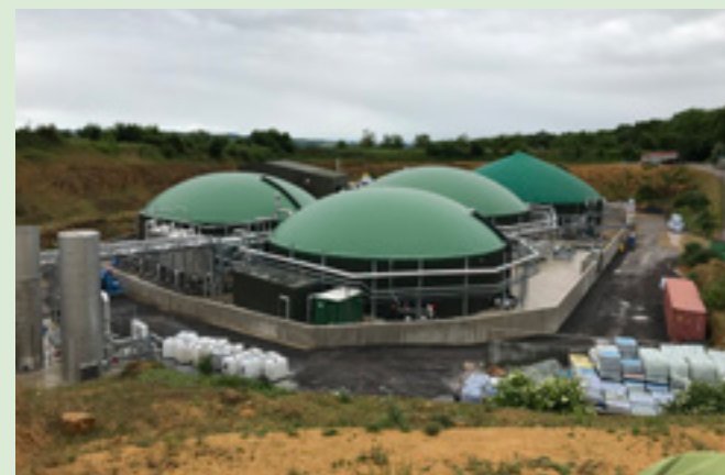
Anaerobic digestion plant
