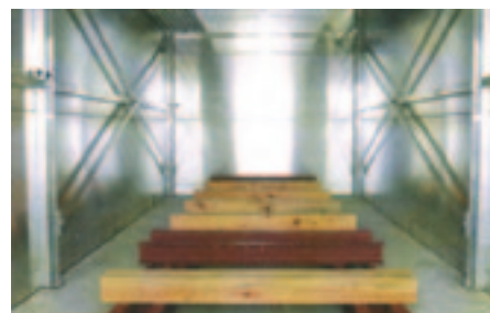
Interior of the kiln showing the heat exchangers and intermediate ceilings
